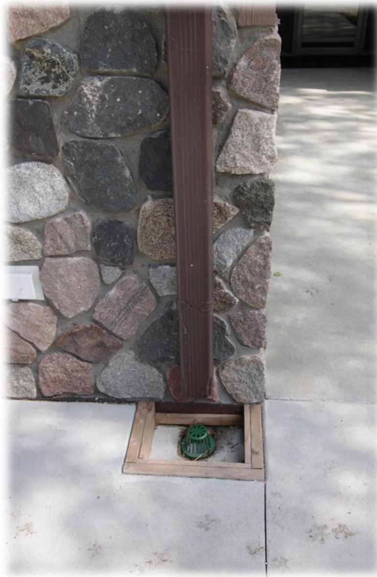
Figure 13. Sub-Surface Drains System
